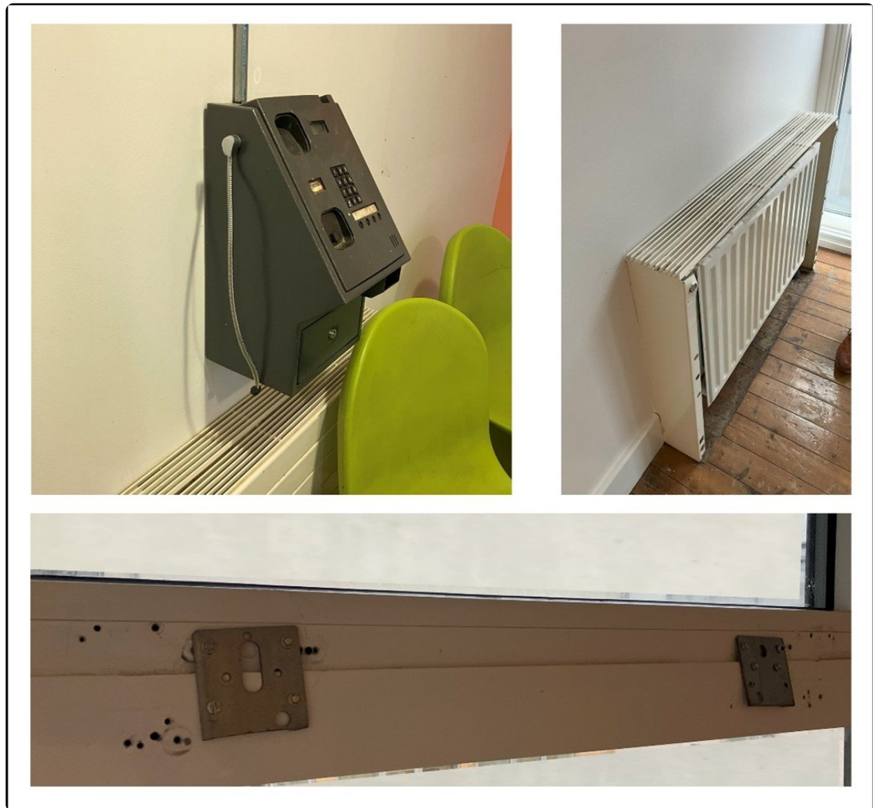
Figure 3 Pictures showing examples of hazards created by fixtures on mental health inpatient wards (pictures: investigation's own). Broken telephone (top left), radiator (top right) and maintenance to securely close a window (bottom)
